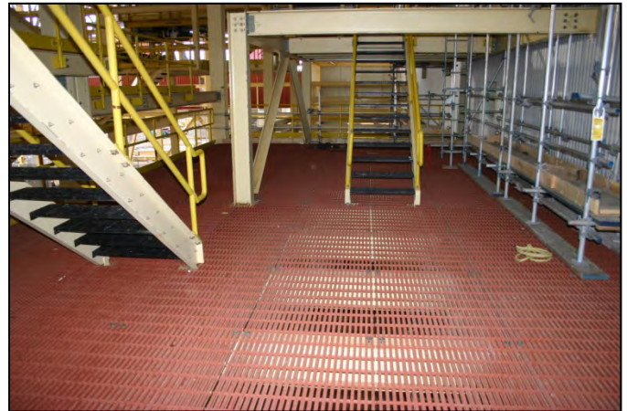
Pultruded Grating used as flooring extensively throughout the plant
